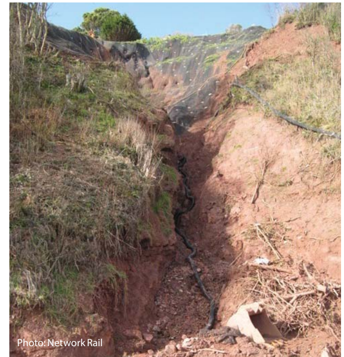
Unstable sandstone cliffs above the line near Dawlish
