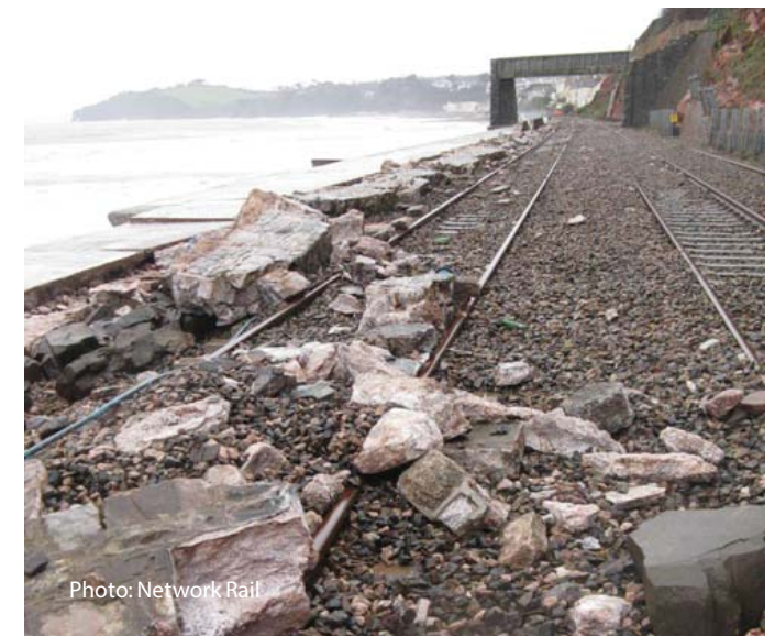
Damage following the February 2014 storms at Dawlish
